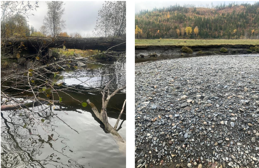
Figure 21. Left: Dilapidated bridge at opportunity 7. Right: Eroding banks and livestock access of opportunity.
