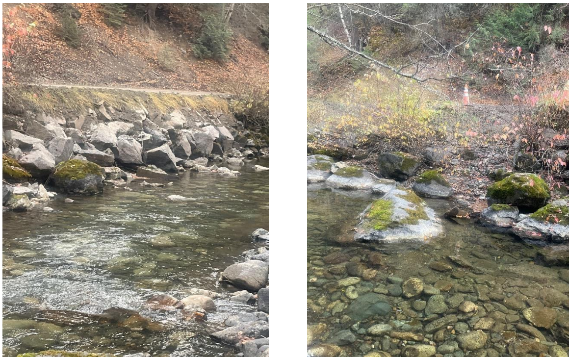
Figure 7. Left: The severe bank steepness along the road has prevented riparian vegetation from taking hold and resulted in riprap collapsing into the stream. Right: A pylon demarks risk to motorists where the road is collapsing into the stream.
