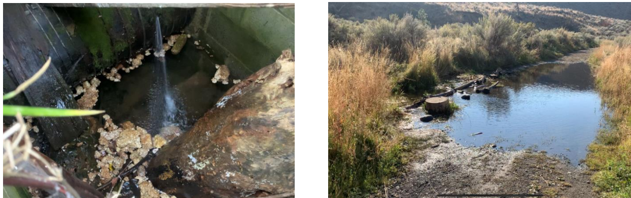
Figure 13. Left: Several leaks are obvious in an exposed section of pipe. Right: Leaking water has pooled in several locations and created artificial wetlands that are not connected to the river.
